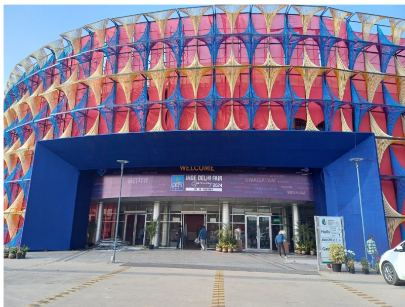
PHOTO – 5 & 6 - Overview of 57th IHGF Delhi Fair Spring'24 - Construction is in full swing at India Expo Mart, Greater Noida.
